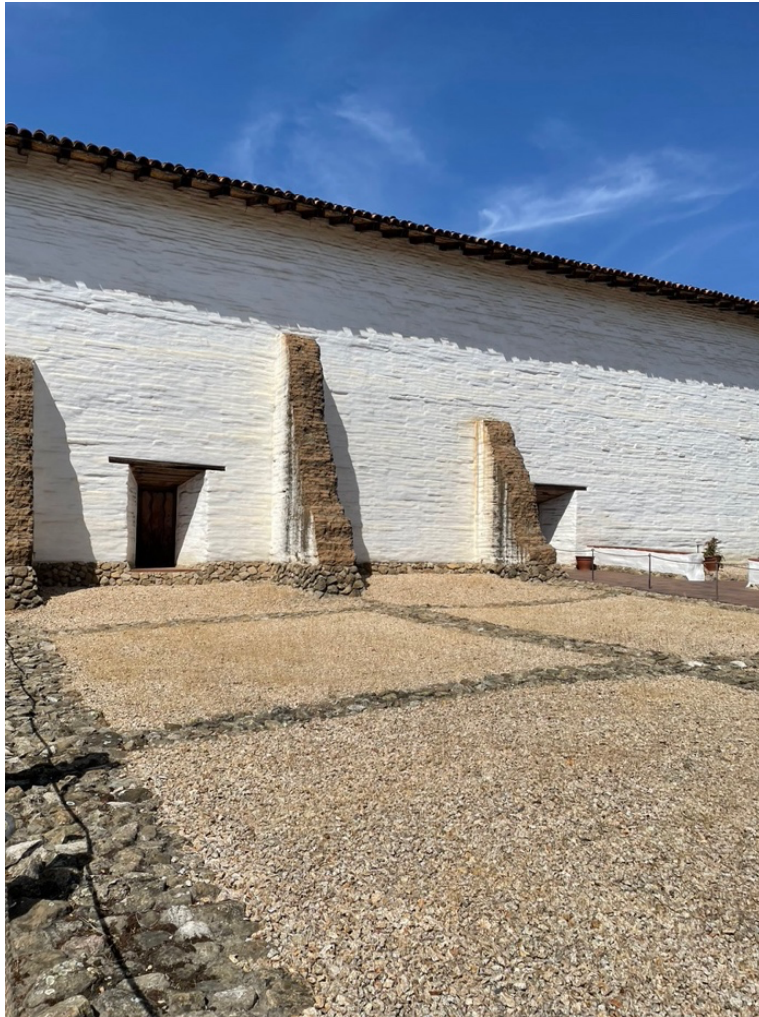
Figure 21. Photograph of south facing wall of the Mission San Jose church with painted and exposed adobe brick. Photograph taken by Lili Flores Aguilar, April 8, 2022.
