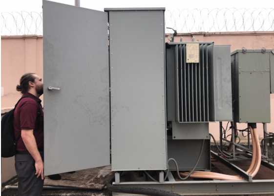
(b) An HV transformer
