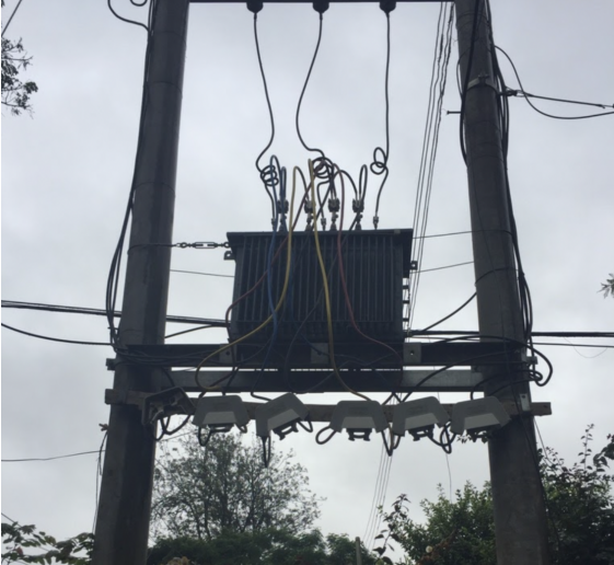
(c) A 3-phase LV transformer
