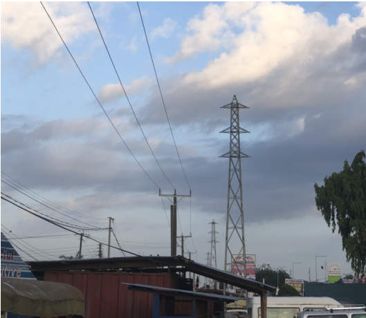
(a) LV, MV, and future HV lines
