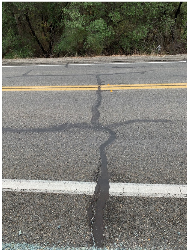
Figure 2.2: Transverse and block cracking.
