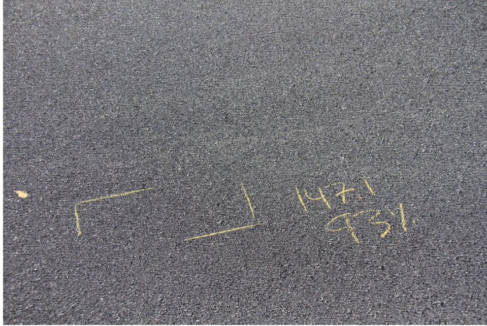
Figure 5.10: Close-up of compacted surface at density test location showing good characteristics and no evidence of segregation.
