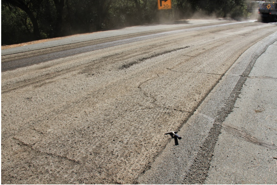
Figure 5.2: Cracking in remaining asphalt after milling.
