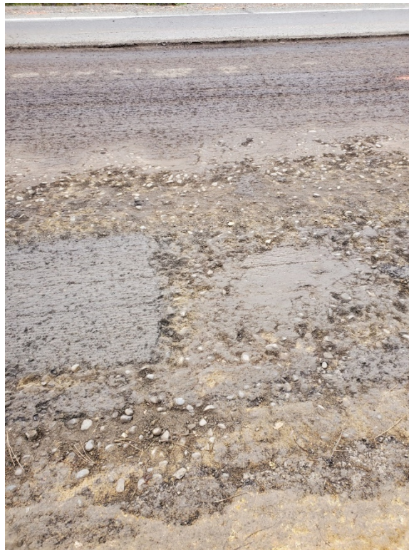
Figure 5.1: Remnants of digouts remaining in asphalt after milling and milling down to aggregate base in half of the lane.
