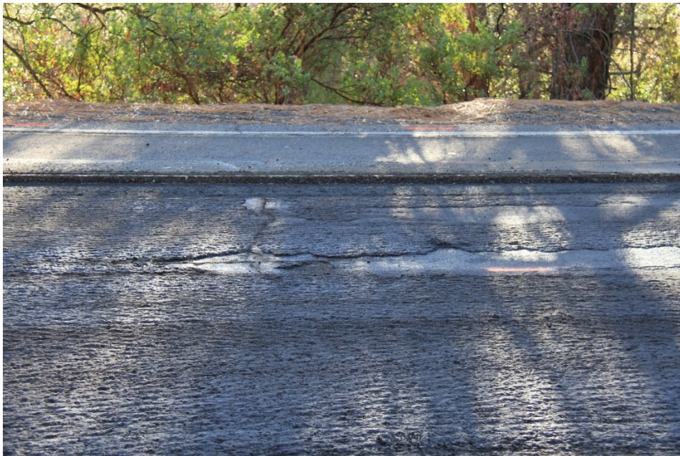
Figure 5.3: Cracking in remaining asphalt after milling.
