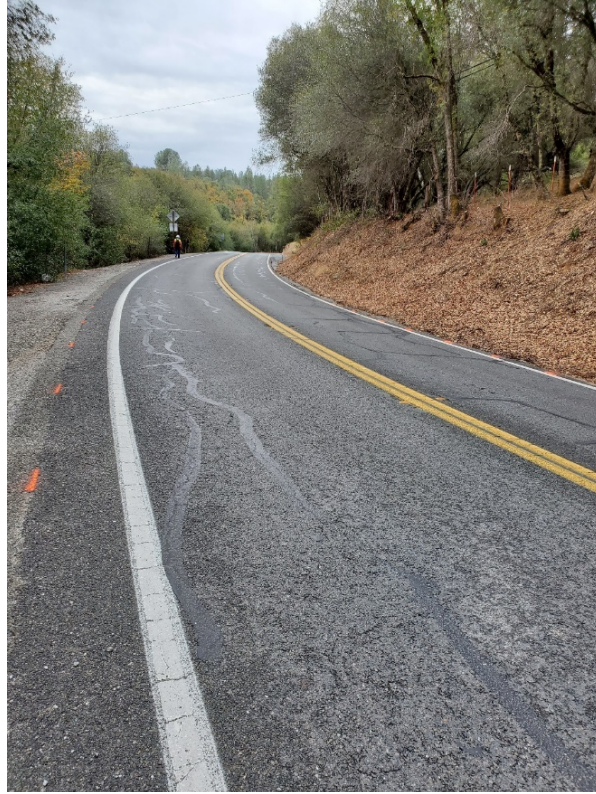
Figure 2.1: Fatigue cracking in the wheelpaths, partly sealed with crack sealant.
