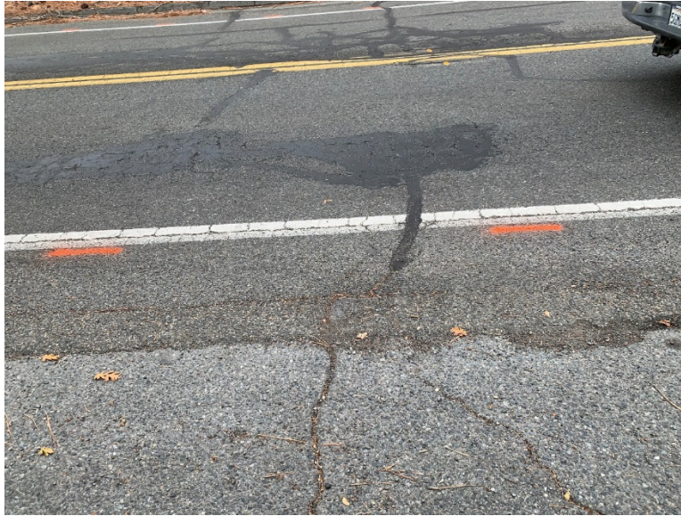
Figure 2.3: Fatigue cracking in the wheelpath and extensive crack sealing.
