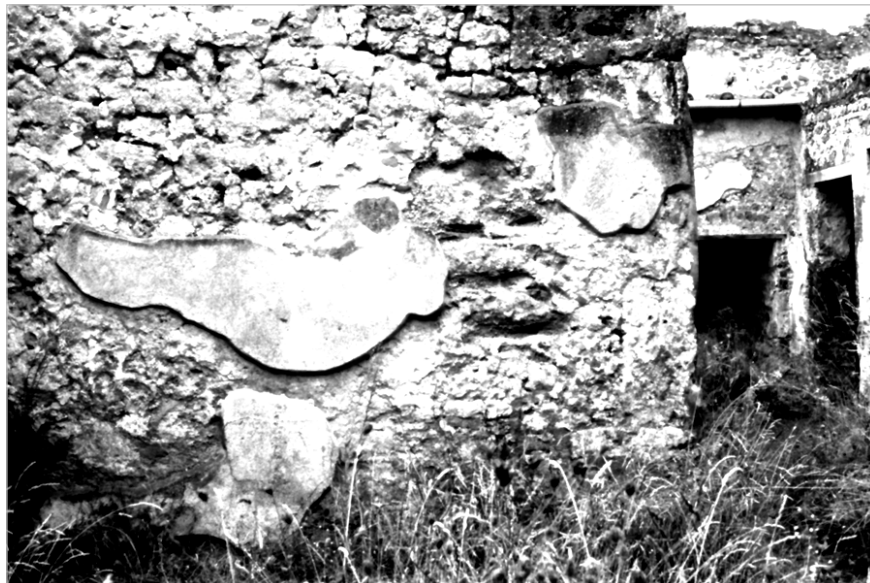
Figure 8.2 South wall of front hall A'' showing hole through to front hall A', with volcanic deposit in situ, Casa dell'Efebo
