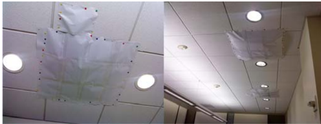
Figure 6.12: The supply air inlet of VAV201 was artificially blocked to simulate a stuck damper.
