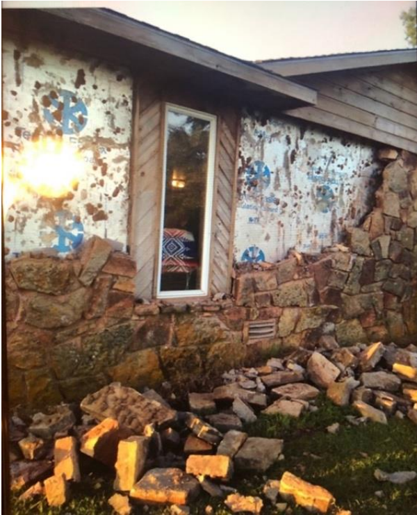
Exterior damages after the M5.8 IE in Pawnee, Oklahoma
