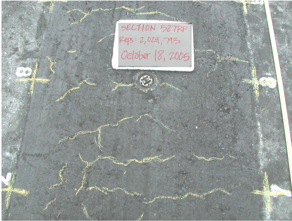
Figure 3.37: Surface cracks marked with crayon between Stations 7 and 8 at end of test.
