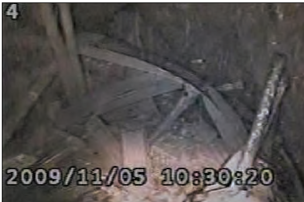
Figure 5.4.3.4.1-1 Blockage in the #5 Shaft 500 ft (152 m) below the collar. [SDSTA]
