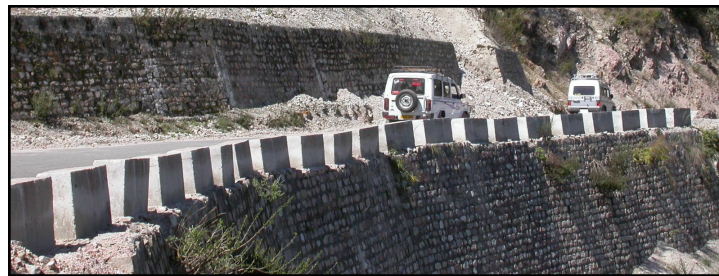
Figure 6. Early failure of toe wall due to heavy precipitation during monsoon (July-August) on NH-58.
