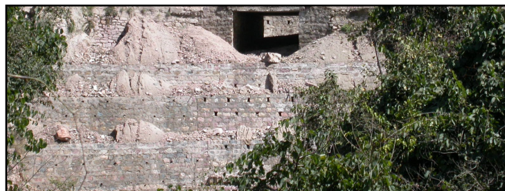
Figure 7. Construction of big culverts and check dams along NH-58 for proper drainage.
