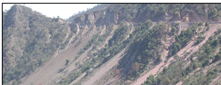
Figure 1. Disposal of cut material downhill into the Alaknanda River caused by the widening activities on NH-58.
