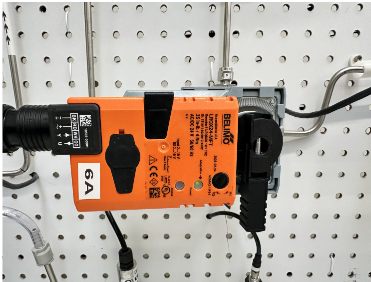
Figure 3.20: Photo of a Belimo 3-way valve on ZeoDe
