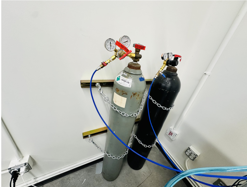
Figure 3.41: Photo of ZeoDe, highlighting the CO_2 and Nitrogen cylinders, and how they are secured to the wall through a two-chain system to a bar that is adhered to the metal struts of the building
