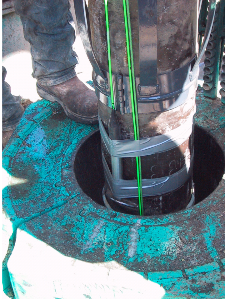
Figure 2.3: As the inner casing was lowered into the well, the fiber cables were strapped to the exterior of the inner casing to hold form and tension until cement was pumped into the annular region. In this photo, we display a lower splice housing for a shallower strain sensor and two fiber cables going to deeper strain sensors. Also visible is a casing “centralizer”. These devices were periodically attached along the casing, typically every 2-3 pipe segments, to keep the cables from pinching between the walls of the inner and outer casings. Not shown are overhead sheaves through which the cables are routed upward and then to the motorized spools that provide nonzero backtension throughout the deployment.
