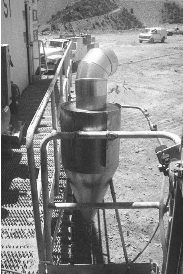
Figure 4b. Dust/cutting collection system installed on a drill rig.
