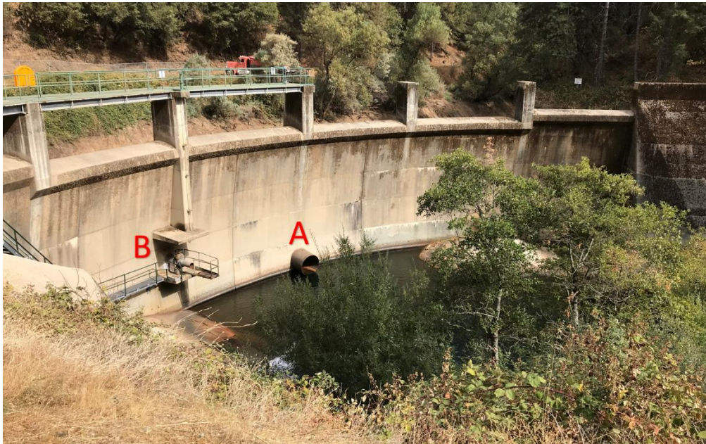
Figure 2.3. Log Cabin Dam. A: Low-Level outlet in LCD site (Diameter: 1.5 m). B: fish outlet for the environmental flow release.
