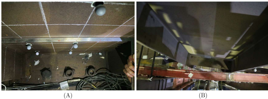
Figure 3.15: Column state at the end of HS-A4: (A) Column base; (B) Second story twisting.
