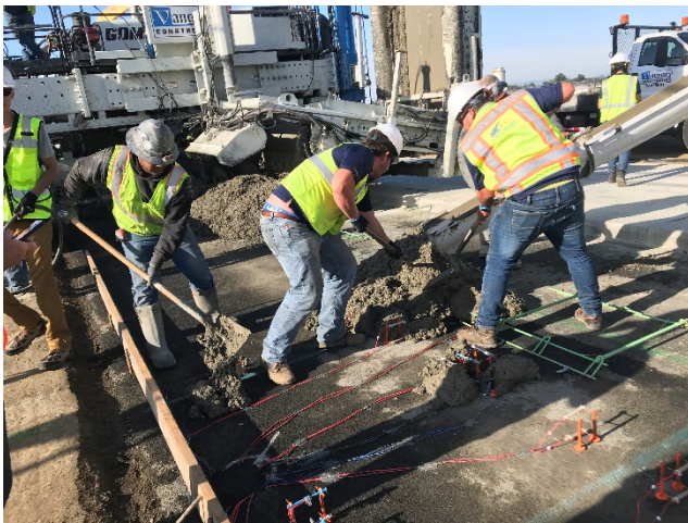
A UCPRC crew shovels concrete around the sensors; then uses the shovels to protect them from the direct impact of the concrete poured from the truck's discharge chute
