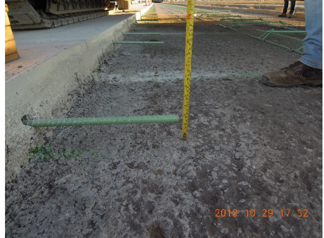
Air pocket around the manually inserted tie bar
