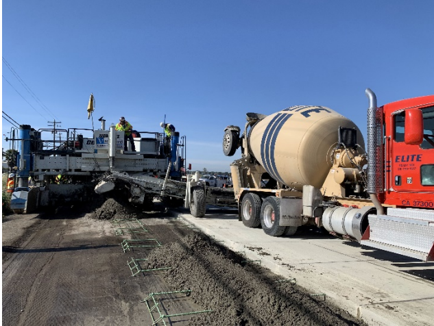
The ready-mix trucks discharge concrete on the belt, then the belt pours the concrete onto the lane. Finally, the spreader spreads the concrete over the width of the lane.
