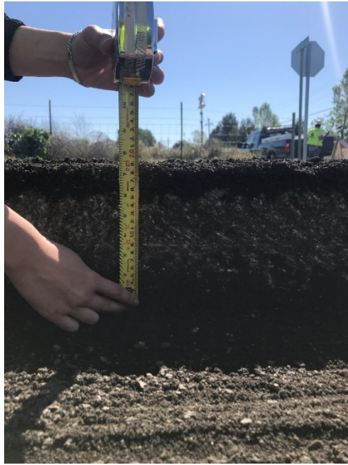
Figure 4.2: Milled asphalt thickness deeper than the 6 in. target value.
