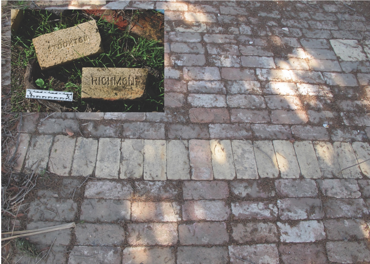
Figure 2.6 This close-up of Pat and Carrie's brick floor shows two different kinds of brick, red and yellow, used to create a precisely laid flat floor. Close ups of similar bricks found at the Bulb show makers marks from the Stockton and Richmond brick companies (inset). (Image credit: the author)
