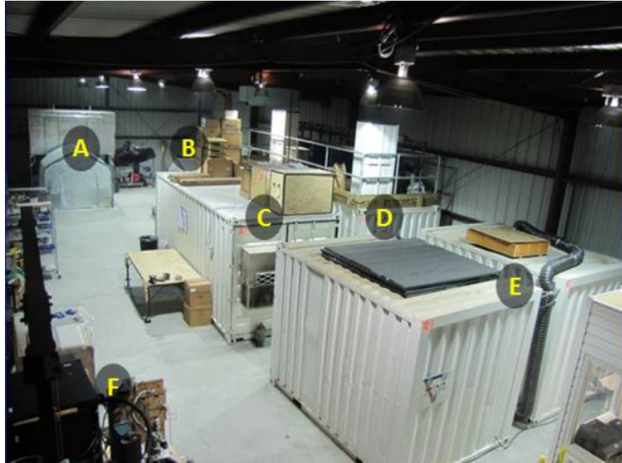
Figure 7.2: A picture of the inside of the KURF scientific facility. The MARS deployment platform was parked at location B.
