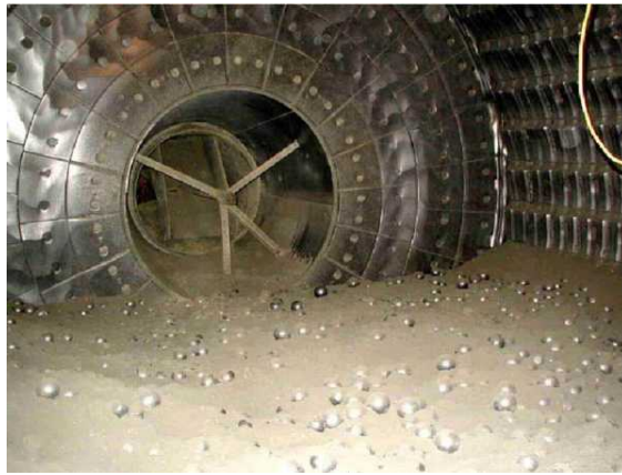
Steel grinding media interspersed with clinker in a cement mill, image courtesy Castle Cement, taken from http://www.understanding-cement.com/mill.html
