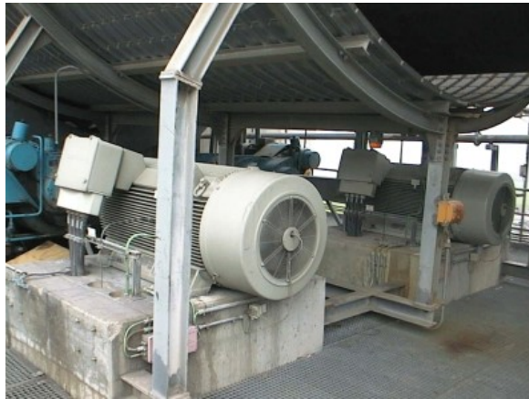
Variable speed drive on cement kiln, image taken from http://fp.is.siemens.de/cement/en/Solutions/Drives_ID.htm
