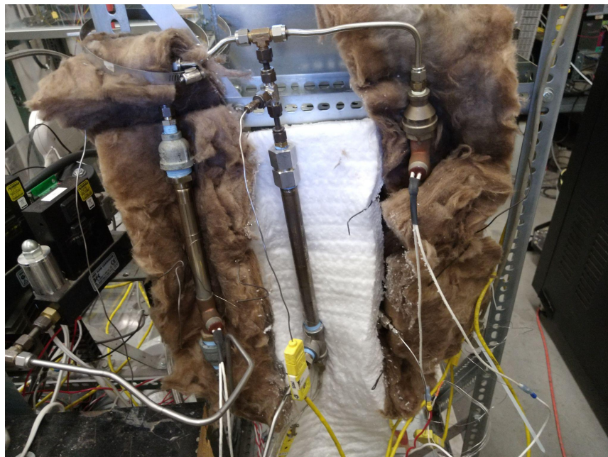
Figure 8. Vaporizers Installed on System
