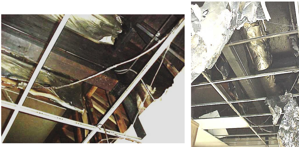
Fig. 22. Fire damages of the Glulam girder (case study).
