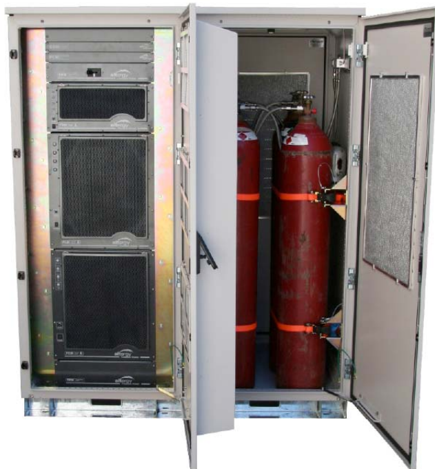
Figure 6: Hydrogen Fuel Cell Cabinet with Hydrogen Supply Cylinders Note: Picture courtesy of Alteryx Corp.
