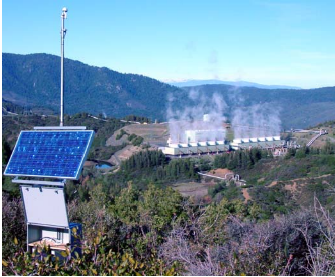
Figure 4-7. Micro-earthquake monitoring station (foreground) and geothermal power plant (background) at the Geysers, California, USA.
