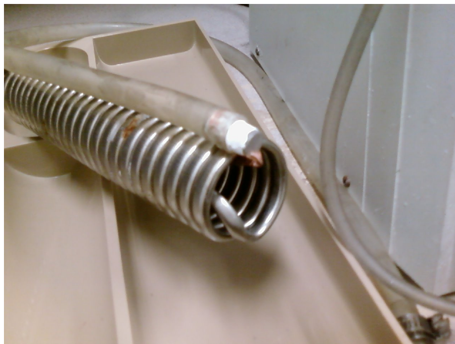
Figure 2.7 – A closeup of the chiller coil and the monel cylinder, attached by the copper sleeve.
