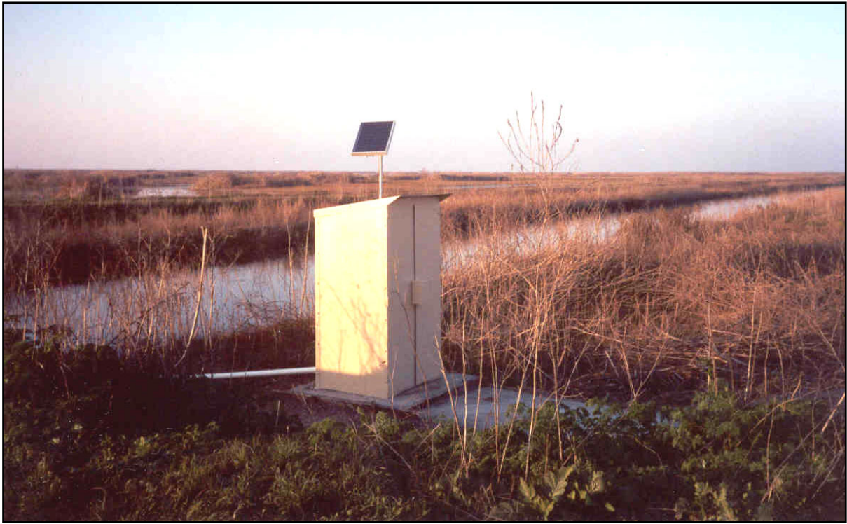
Figure 2.11. Volta Wasteway monitoring station.
