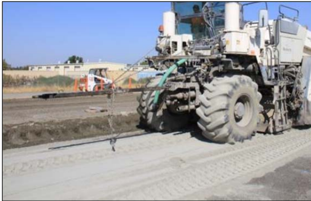
Figure 3.27: FDR-PC: Excess cement on Cell #7.
