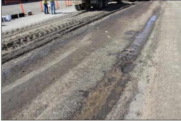
Figure 3.19: FDR-EE: Puddled water on surface after compaction.
