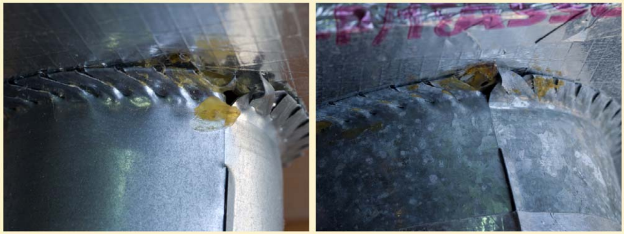
Figure 18 Splitter box starter leak locations
