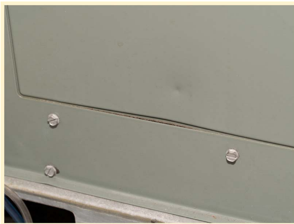
Figure 14. Dent in RTU blower access panel.
