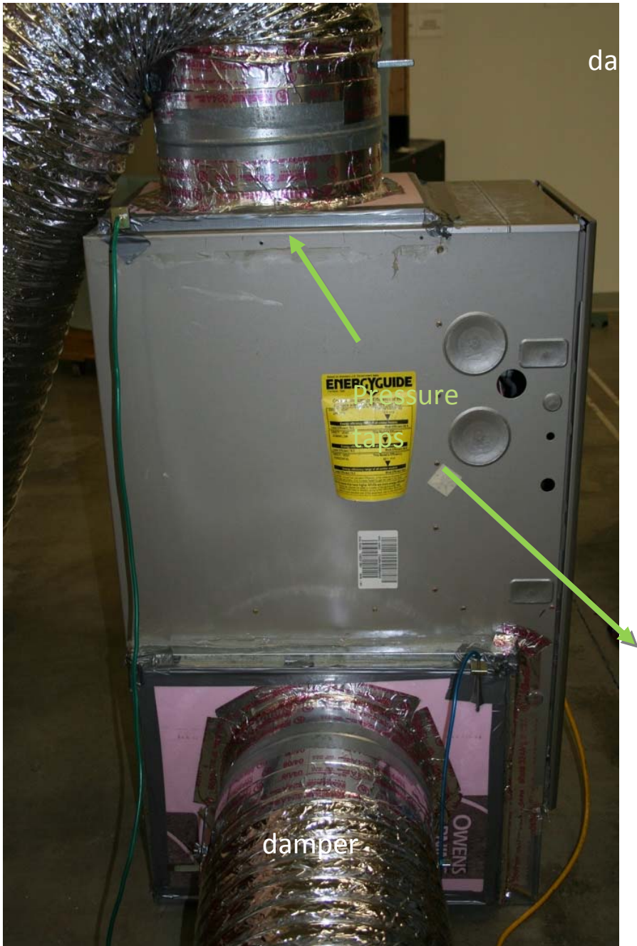
Figure 7. Flex duct and damper mounting on Bryant furnace
