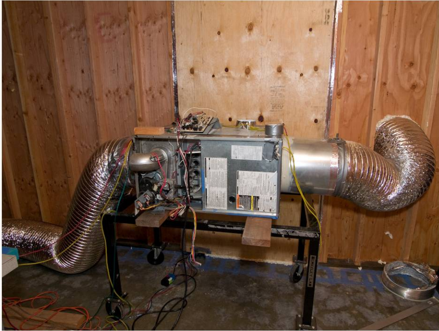
Figure 3. Furnace connected to test chamber with flexible ducting
