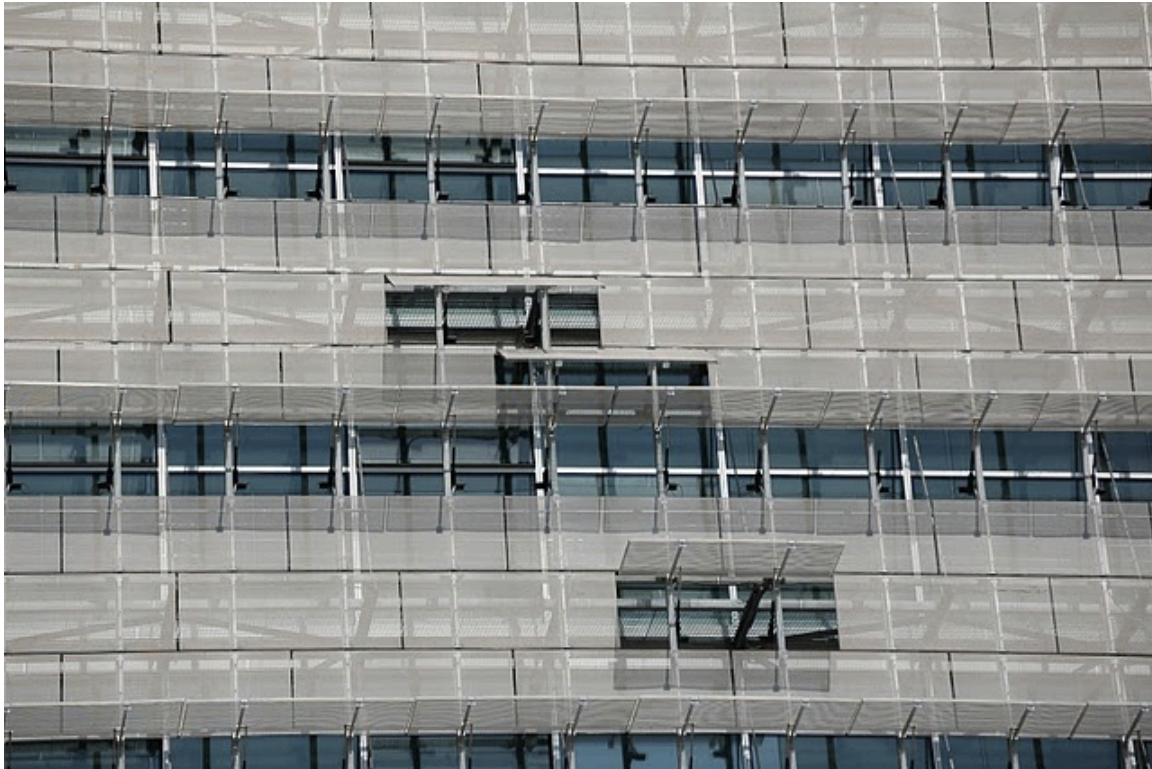
Figure 3.9 Exterior view of the SE exterior metal screen. Image shows select panels that are open. 12
