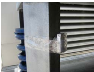
Figure 4.9 Location of exterior rooftop temperature sensor.
