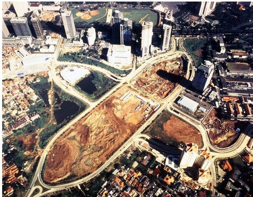
Top: The kampung that was cleared for the development of SCBD, ca. 1987. Bottom: SCBD infrastructure under construction, ca. 1992-1993. Images from scbd.com .
