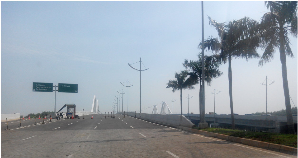
Bridge from Pantai Indah Kapuk (PIK) to Island D, Golf Island, under development by PT Kapuk Naga Indah, subsidiary of PT Sedayu Group. Image by author, 2015.
