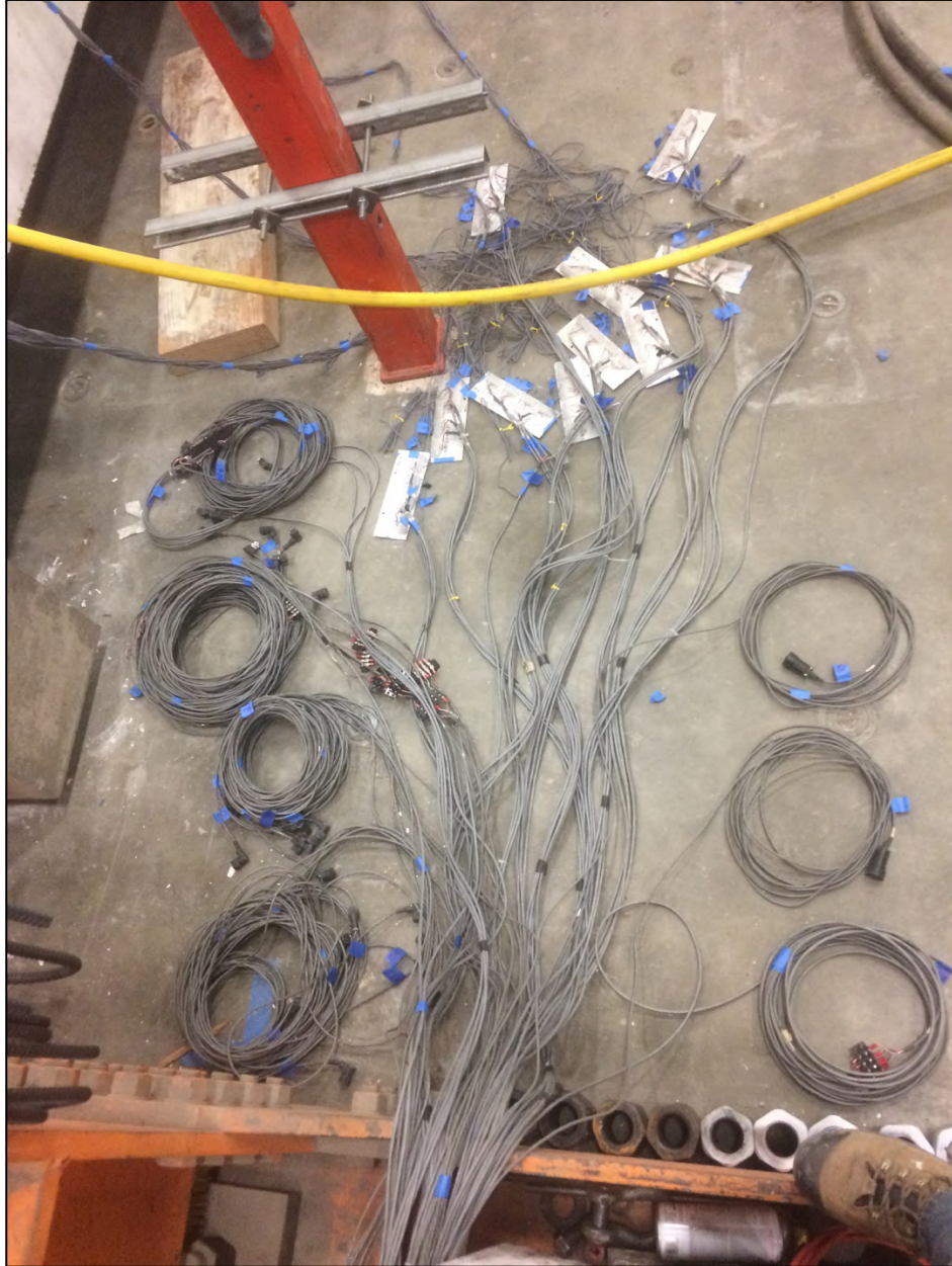
Figure G- 35. Instrumentation cable management
