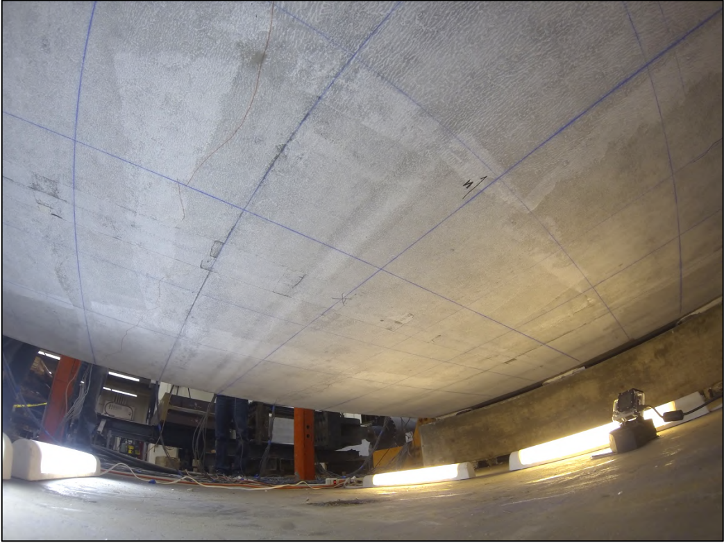
Figure 5-6. Minimal damage observed on specimen bottom surface as seen from the east
