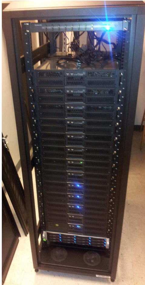
Figure C.1: Server rack containing the Excelso cluster and Calypso fileserver.
