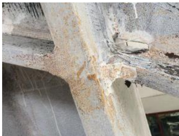
(b) Closure of Fractures at Beam Bottom Flange Level
