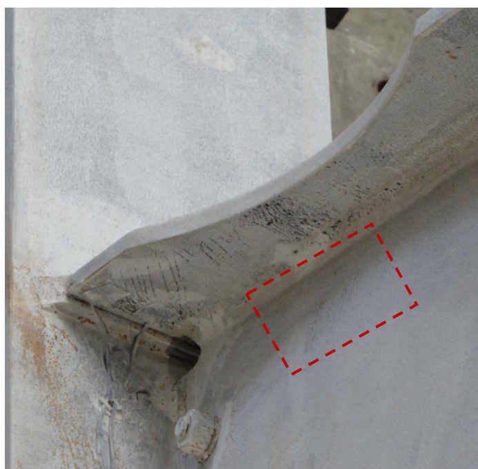
(b) Detail A, Yielding on Beam Web
