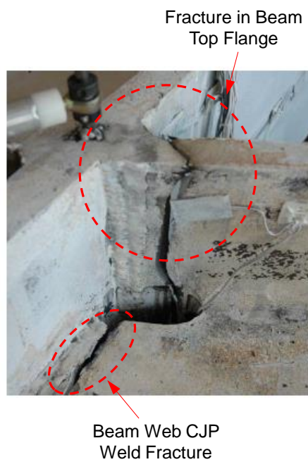
(b) Close-up View of The Fracture
