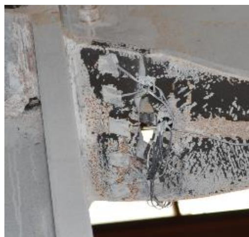
(c) Beam Bottom Flange Fracture
