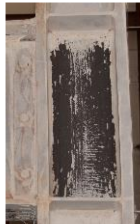
(f) Detail D, Significant Panel Zone Yielding and Column Kinking
