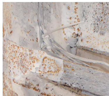
(b) Detail A, Minor Crack at End of Beam Web CJP Weld
