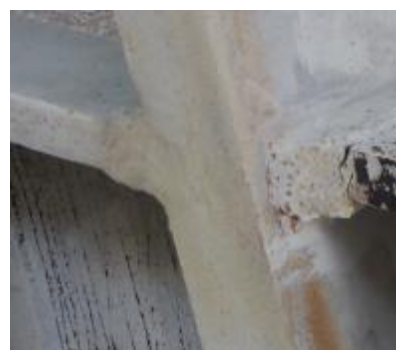
(c) Detail B, Minor Beam Top Flange CJP Weld Crack
