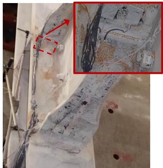
(c) Column Flange Yielding Due to Column Kinking (Front Side)
