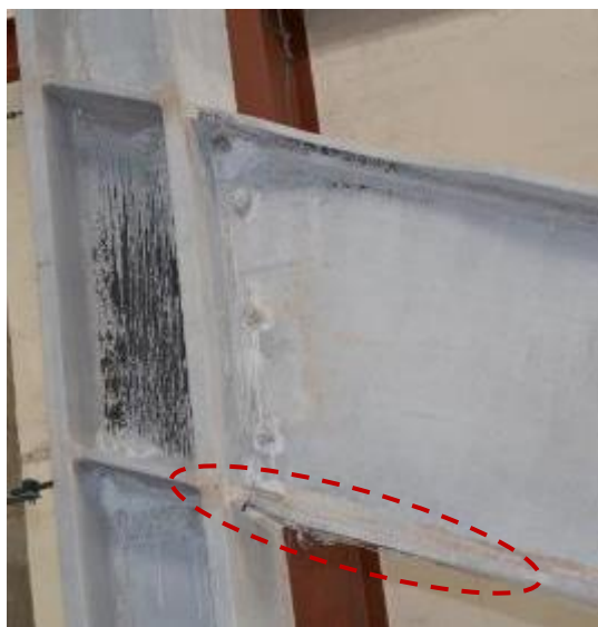
(a) Minor Beam Flange Local Buckling
