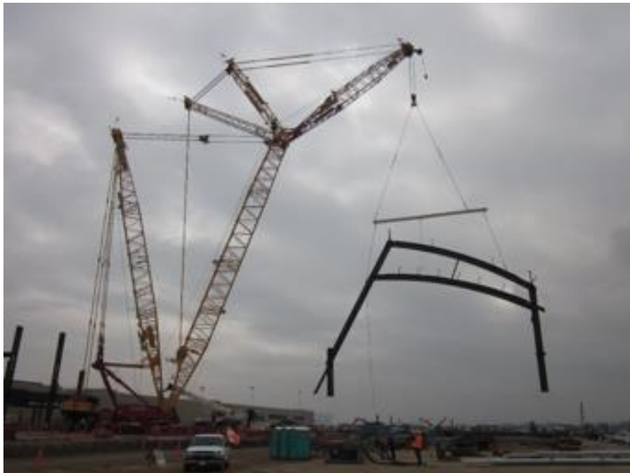
Figure 5.6 Erection of SMF with Sloped Connections (courtesy of T. Kuznik, The Herrick Corporation)
