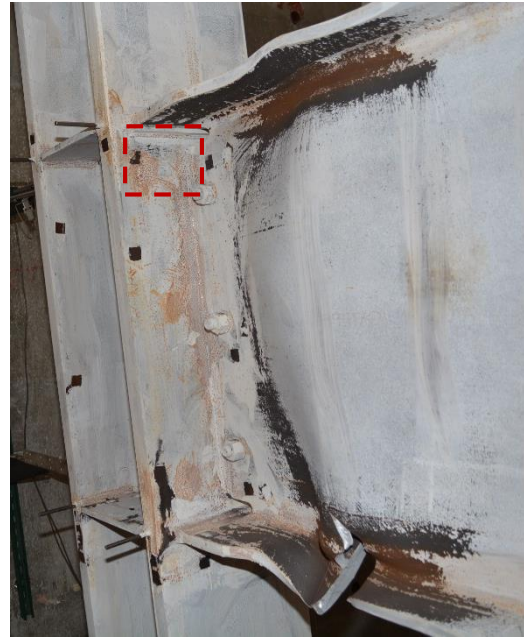
(c) Column Flange Yielding Due to Column Kinking (Front Side)
