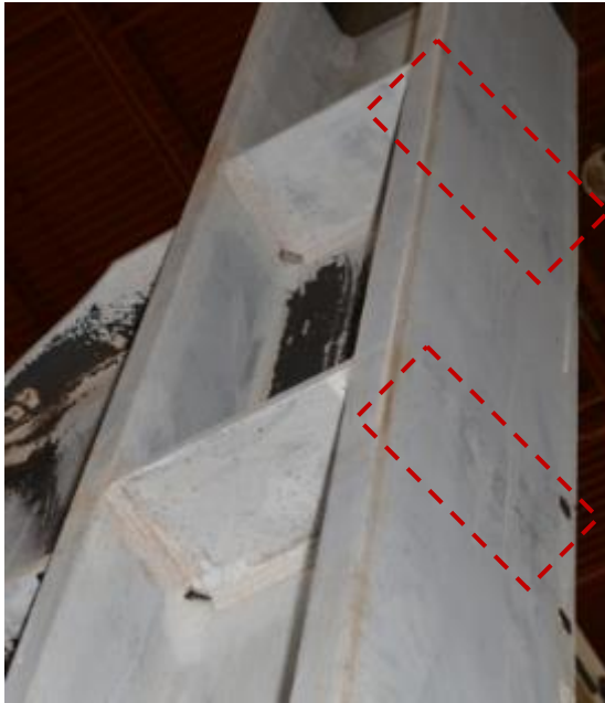
(b) Column Flange Yielding Due to Column Kinking (Back Side)
