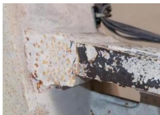
(c) Detail B, Minor Beam Top Flange CJP Weld Crack
