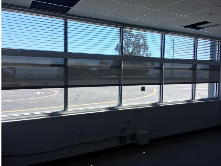
Figure 4. Internal view of FLEXLAB testbed with INTER shading system installed
