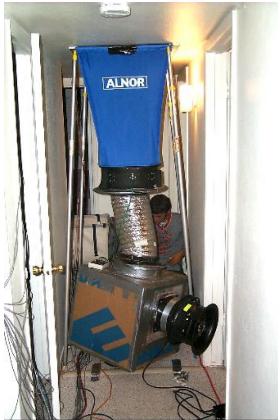
Figure B6. Multiple fan-flowmeter return powered flow hood
