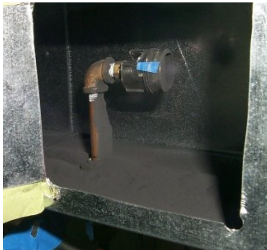
Figure D3. Dust deposited on filter mount and duct wall
