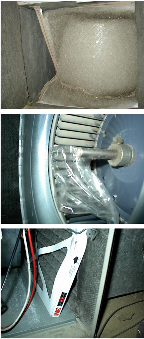
Figure 13. Filter bypass examples: filter wrapped around fan, bag bypassed filter into fan blades, wrong size filter forced into filter slot (the first photograph is from Paul Francisco of Ecotope)
