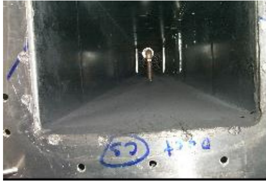
Figure D1. Deposition on filter rack and duct walls upstream of the coil
