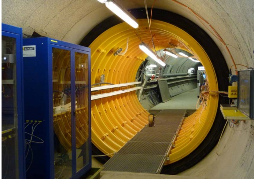
Figure 5-1. Tunnel packer system used to isolate the MI shear zone. Small disks with tubing issuing from them (inside yellow packer) are “surface packers” that seal the tunnel wall and collect water from inflow points. Tunnel diameter is 3.5 meters.
