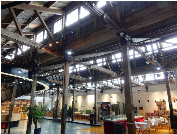
Figure 3- 7 Images of the roof inside of the Workmanship Demonstration Pavilion Museum. Photography by the author.
