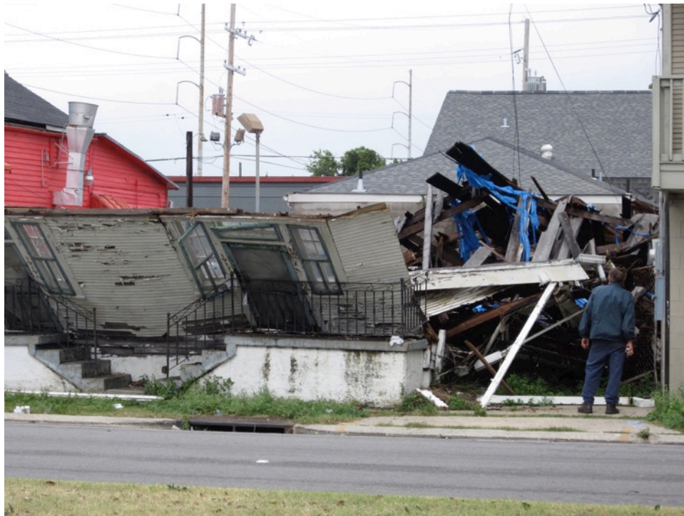
Figure 4. Collapsed house. Photo by author. 2012.
