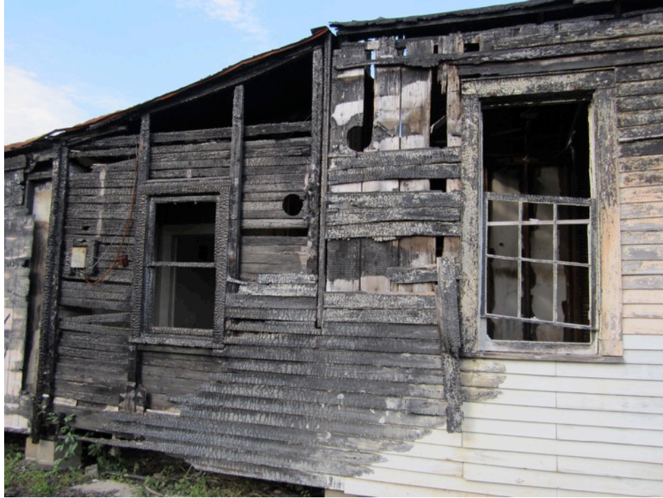
Figure 21. The fire-damaged rear of the house. Photo by author. 2013.
