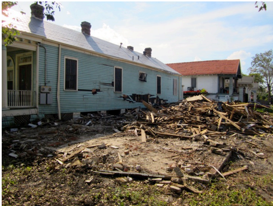
Figure 12. The remains of a collapsed house. Photo by author. 2012.
