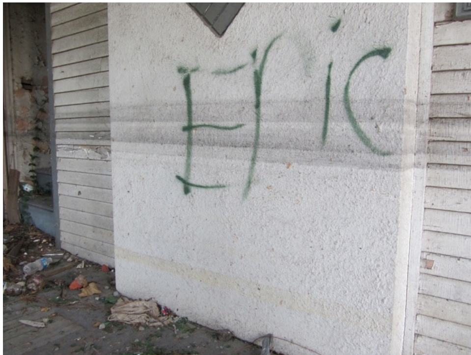
Figure 13. Water lines still visible on a house in Mid-City. Photo by author. 2012.
