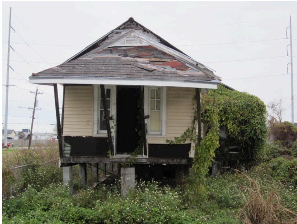
Figure 26. A property in “very poor” condition. Photo by author. 2013.
