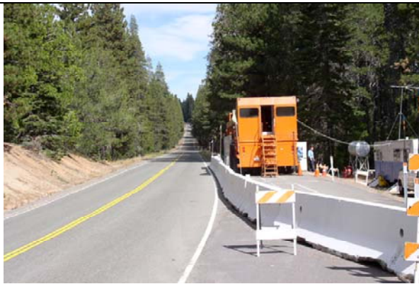
HVS2 on SR-89 foamed asphalt test sections, Calpine, California, fall 2003.
