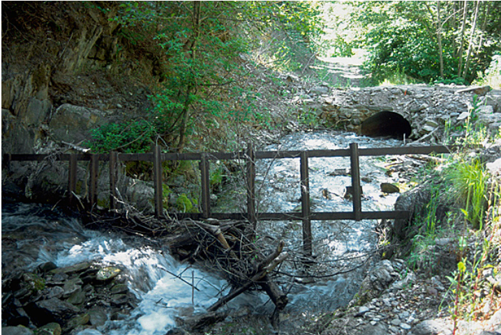
Figure 24. A trash rack installed upstream to protect a culvert from plugging. Source: Keller and Sherar 2003.
