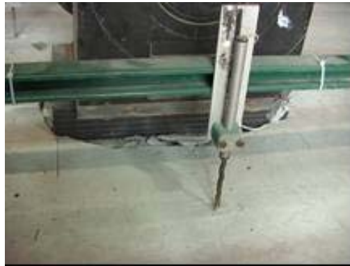
Figure 5.55 Punch-through of the load through concrete at top of slabs
