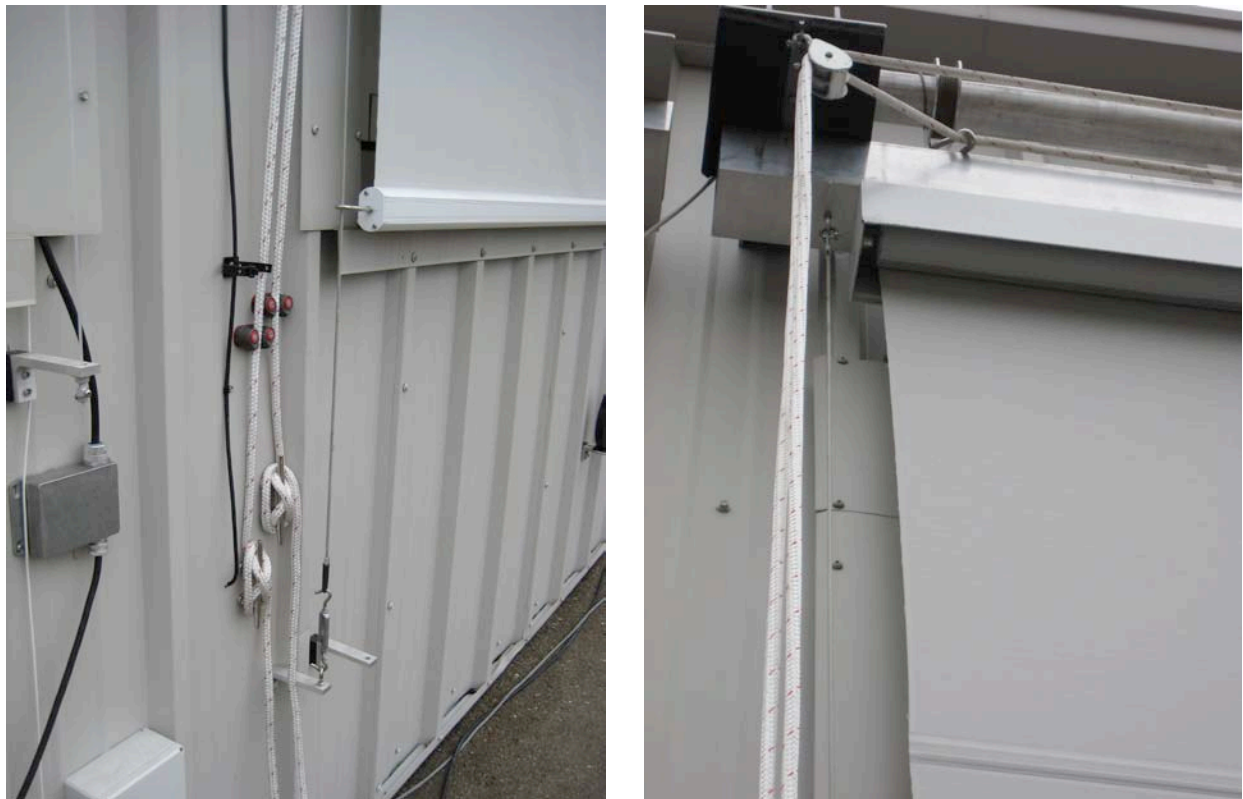
Figure 30: Views of lower hem bar (left) and header (right) mounted on the hoist system.
