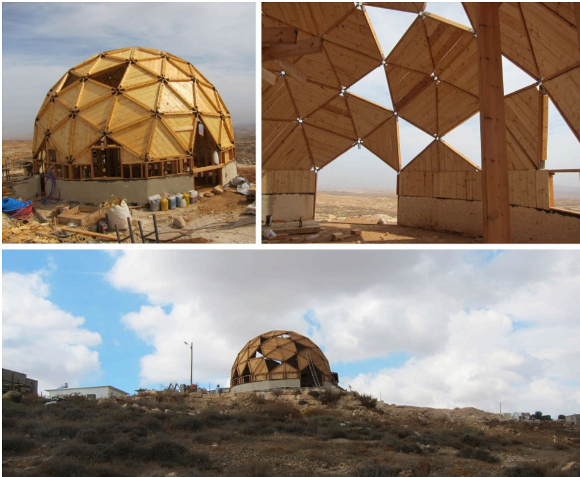
Figure 5.26 Hila and Evyatar’s geodesic dome, 2015. Since the above pictures were taken, Dotan and his team had covered the wooden shell with different materials. Nevertheless, it is still uninhabitable. Photos by the author.
