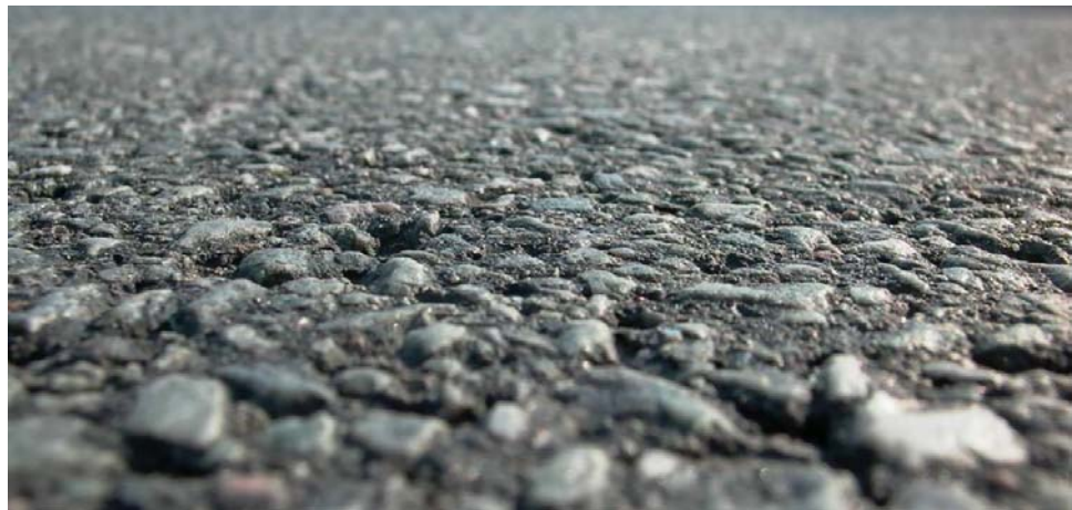
Figure 1.10. A three years old dense-graded asphalt concrete (DGAC) where the bitumen film has been worn off and where no significant signs of wear and tear and distress can be observed.
