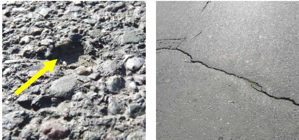
Figure 1.11. Raveling, loss of aggregate (to the left) and cracking (to the right).
