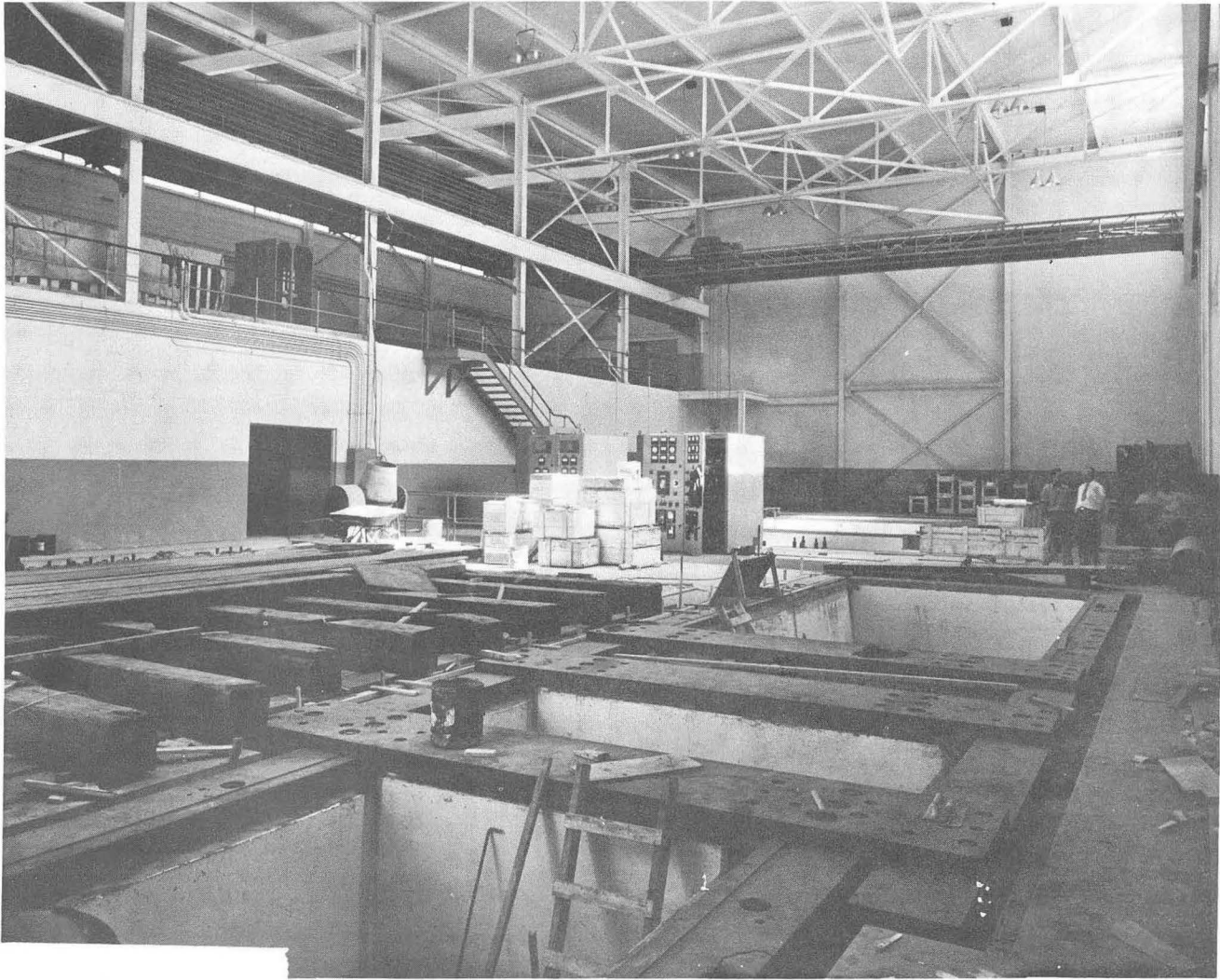
Fig. 11 View from motor end of bed plates upon foundation walls of west machine. Note groove in bed plate for motor stator and generator stator rollers. Planking and shoring of generator room floor was necessary to protect from overloading by heavy machine components.
