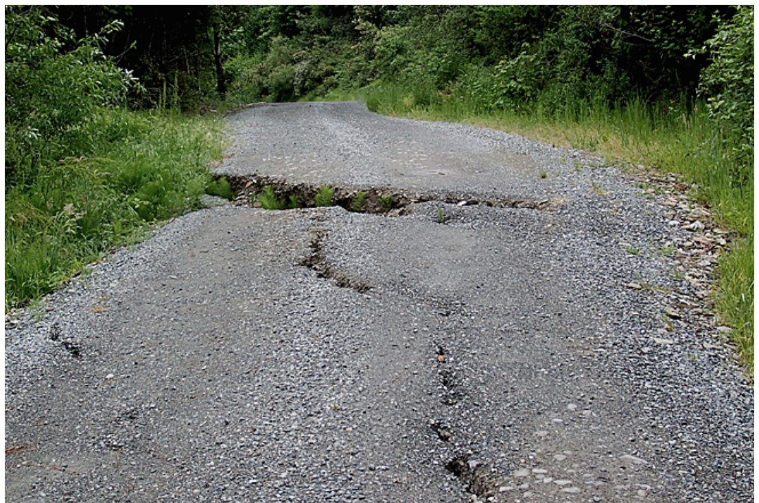
Figure 21. Cracks appearing in the road surface, especially at the edges of fills, are a sure sign of an impending failure or landslide. The horsetail growing in these cracks indicates that the source of the problem is groundwater seeping through the road bed. Photo: Richard Harris.
