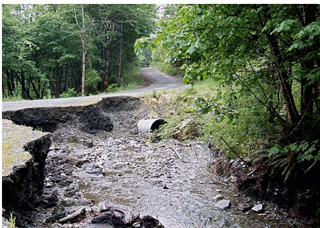
Figure 18. This culvert plugged with debris during a storm. Although it is still in place, the swirling water and debris caused extensive erosion of the road and the adjacent old log landing. This type of failure is common on older “legacy” roads where crossings were not adequately designed to pass 100-year flows plus debris and sediment. In many cases, the culvert will be displaced and transported downstream.
