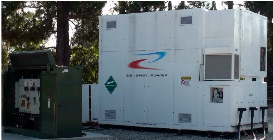
Figure 58: View of the Zenergy Power Medium Voltage distribution-level three-phase Saturated Core FCL operating at Southern California Edison in Avanti Circuit of the Future.
