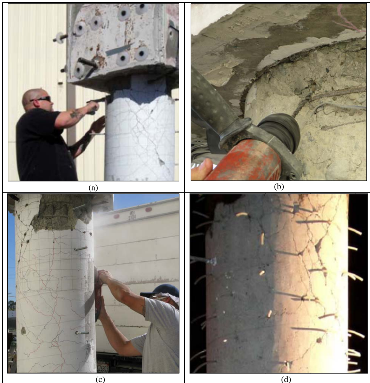
Figure 2.8 Repair of as-built test specimen (preparation stage): (a) hammer test to remove loose material; (b) hole-drilling in the cracked regions; (c) grinding of the surface paint; (d) Injection ports in damaged regions.
