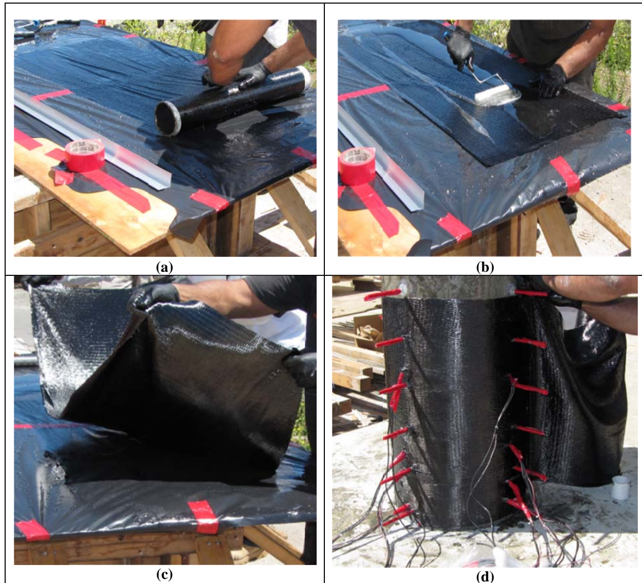
Figure 1.1 Wet layup process: (a) CFRP roll; (b) application of epoxy; (c) CFRP soaked in epoxy resin; (d) wrapping of the column specimens.
