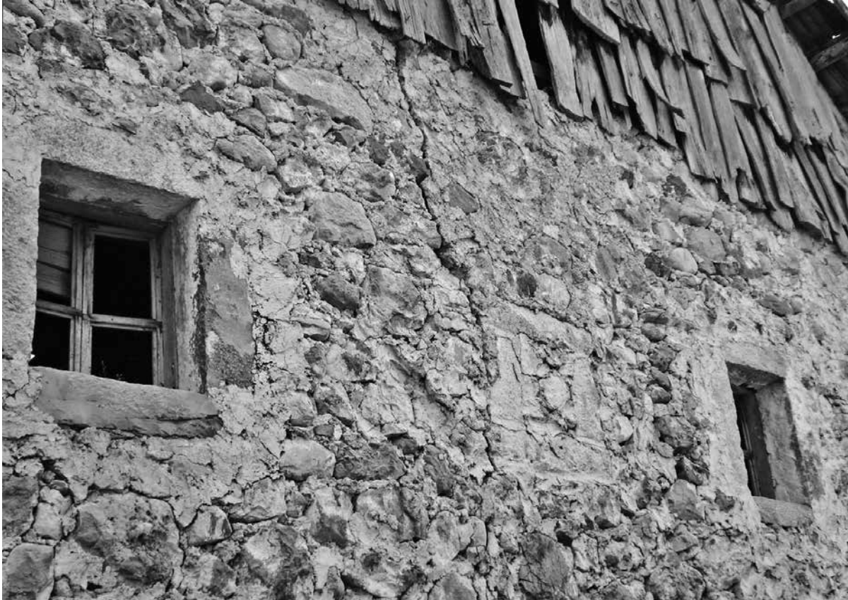
Figure 7.17. Closed frëngji (right) and larger replacement window (left) (ST285, Ndërlysa). Ann Christine Eek
