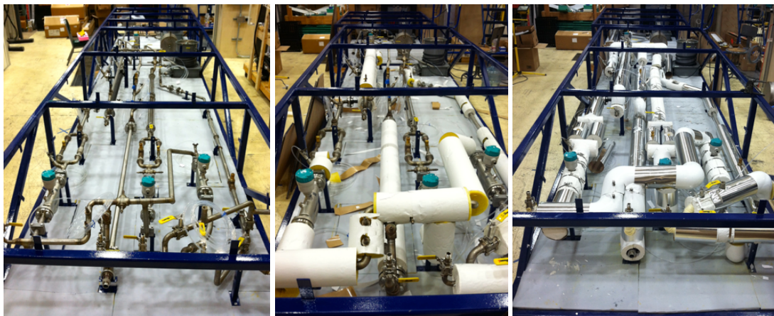
Figure 2-5. CIET 1.0 piping insulation in progress, February 2014 (left), March 2014 (center) and April 2014 (right).
