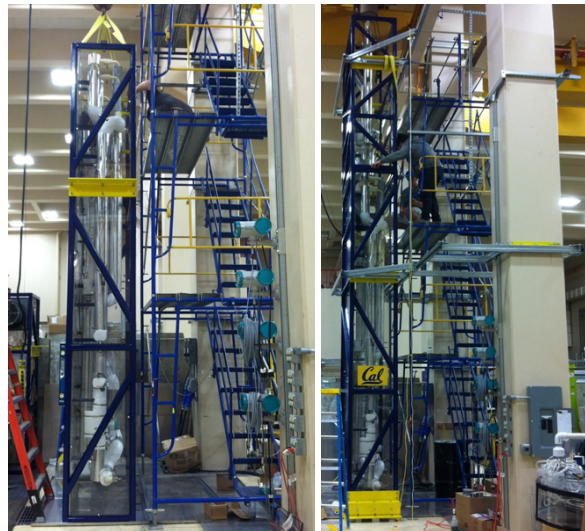
Figure 2-6. CIET 1.0 lower (left) and upper (right) frame assemblies being set in place, June 2014.
