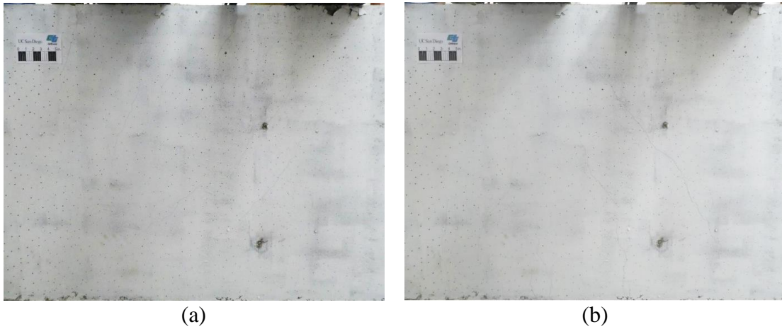
Figure 4.21. Minor Shear Cracking Observed in West Face of Bent Cap Joint at: (a) Peak of Displacement Ductility +4; (b) Peak of Displacement Ductility -4
