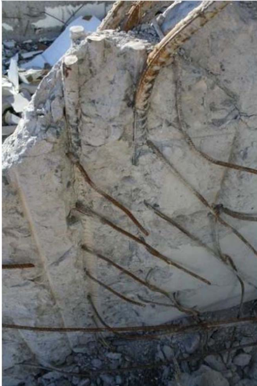
Figure 3.18 - Post-earthquake picture of Axis 8 (after IDIEM, 2010)
