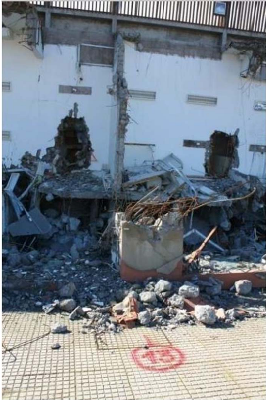
Figure 3.21 - Post-earthquake picture of Axis 13 (after IDIEM, 2010)
