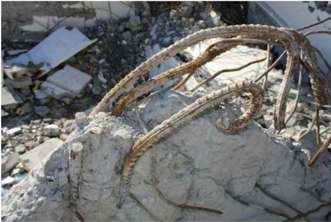
Figure 3.16 - Post-earthquake picture of Axis 8 (after IDIEM, 2010)
