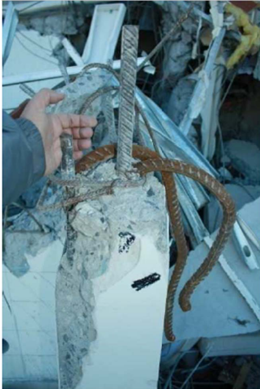
Figure 3.19 - Post-earthquake picture of Axis 11 (after IDIEM, 2010)
