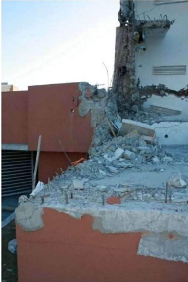
Figure 3.13 - Post-earthquake picture of Axis 5 (after IDIEM, 2010)
