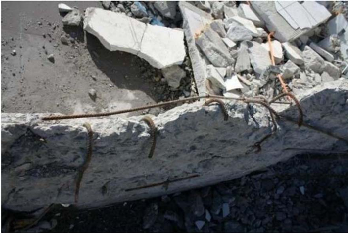
Figure 3.15 - Post-earthquake picture of Axis 8 (after IDIEM, 2010)
