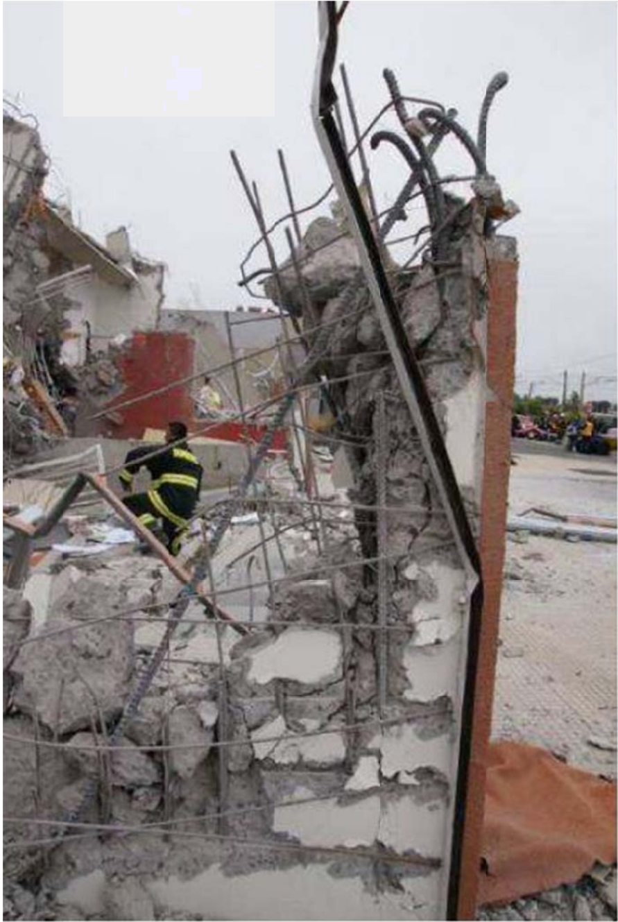
Figure 3.24 - Post-earthquake picture of Axis 13 (after IDIEM, 2010)
