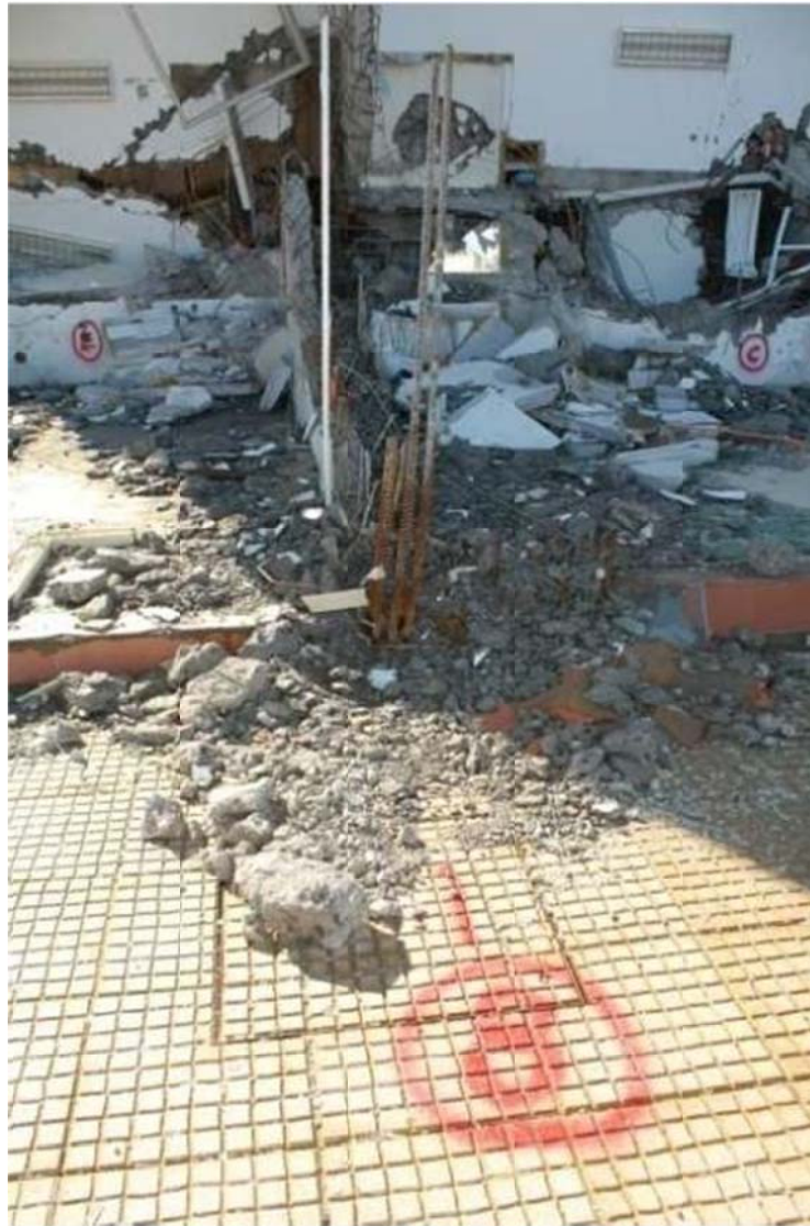
Figure 3.14 - Post-earthquake picture of Axis 8(after IDIEM, 2010)
