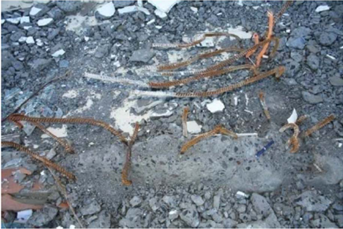
Figure 3.20 - Post-earthquake picture of Axis 11 (after IDIEM, 2010)
