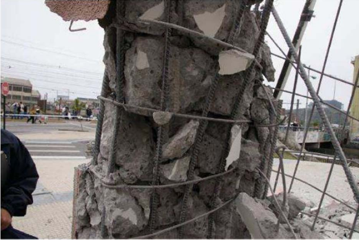
Figure 3.25 - Post-earthquake picture of Axis 13 (after IDIEM, 2010)
