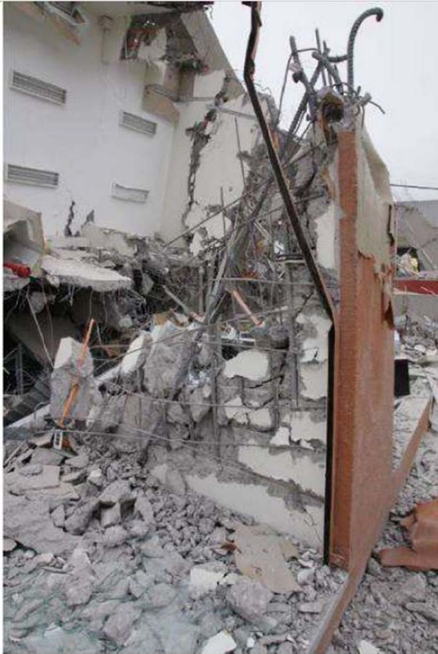
Figure 3.23 - Post-earthquake picture of Axis 13 (after IDIEM, 2010)
