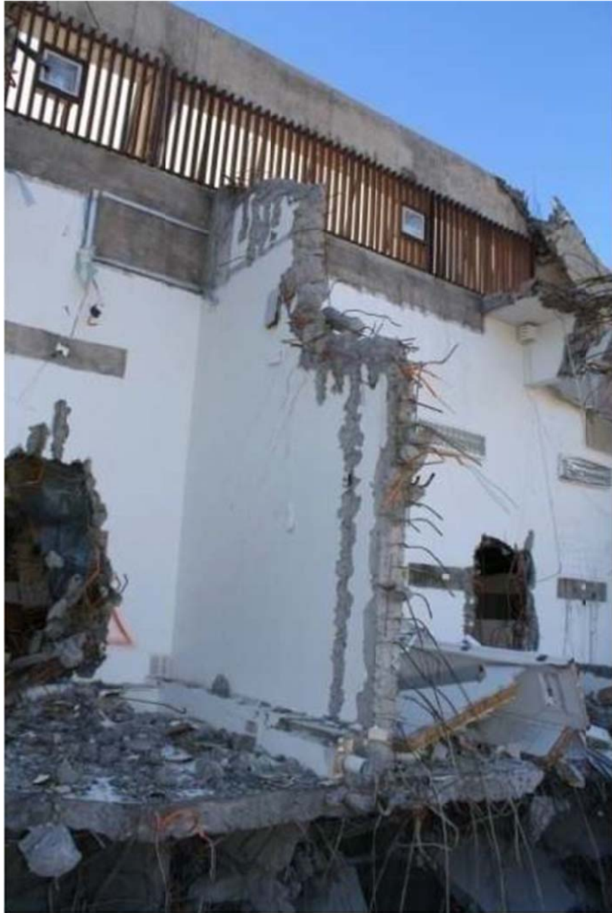
Figure 3.22 - Post-earthquake picture of Axis 13 (after IDIEM, 2010)
