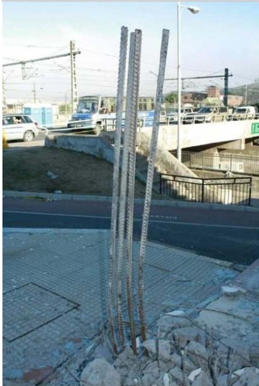
Figure 3.17 - Post-earthquake picture of Axis 8 (after IDIEM, 2010)
